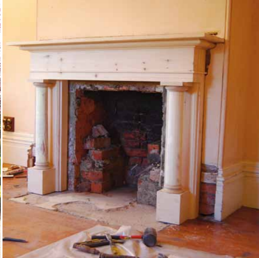
The drawing room mantelpiece in its raw timber state during the restoration
